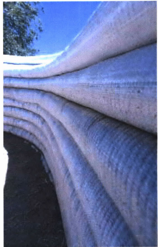
Figure 3 Earthbag construction based on stabilized and compressed earth packaged into polypropylene skin to form continuous bricks: Source: CalEarth Institute
